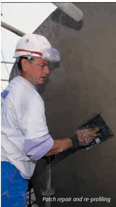
Cathodic protection with titanium mesh
