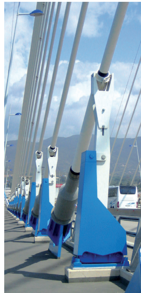
PED damper Charilaos Trikoupis bridge / Greece
