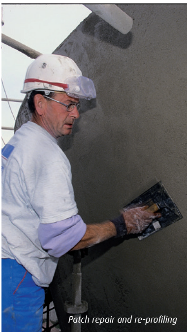
Cathodic protection with titanium mesh
