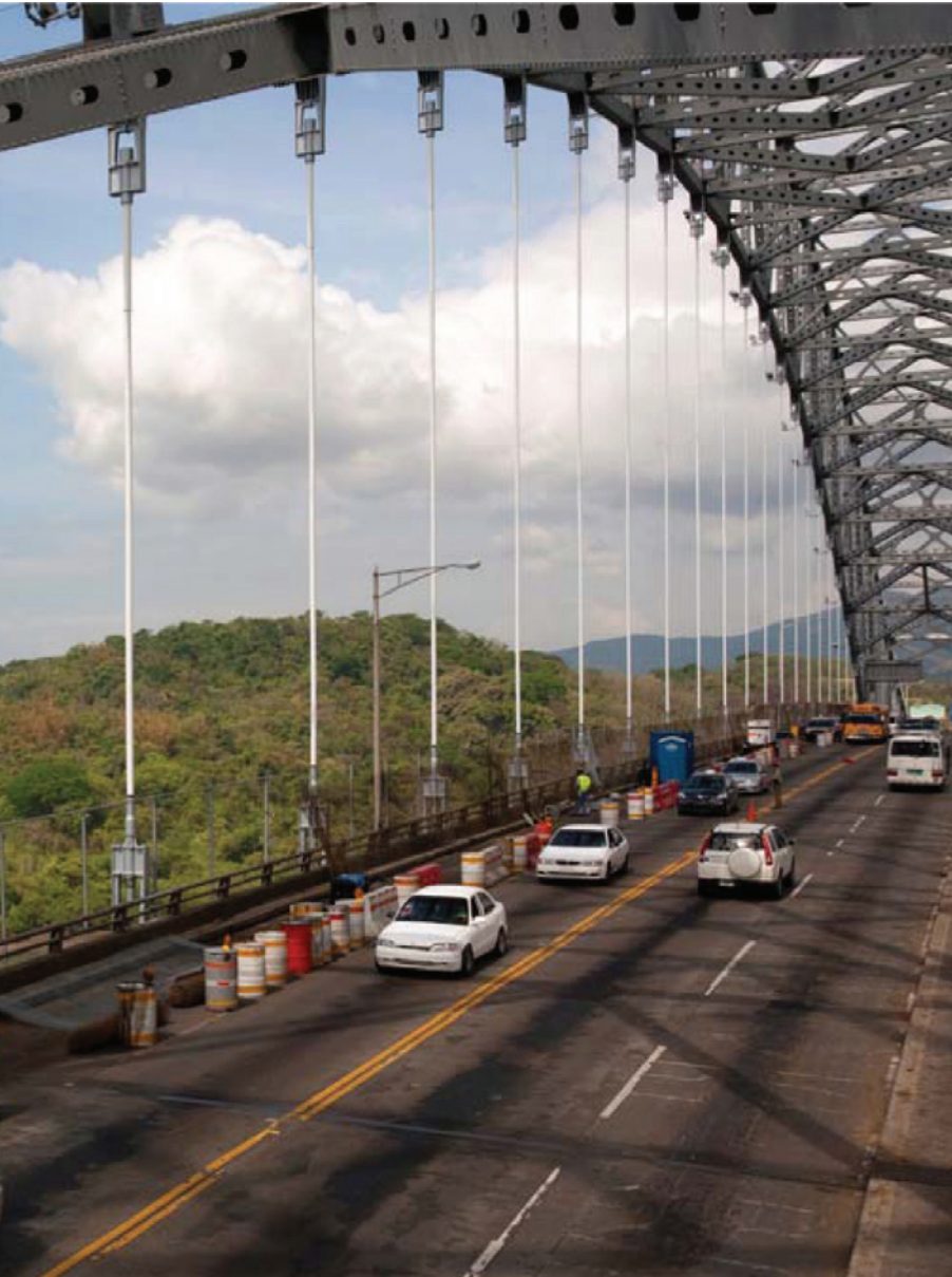
H1000 cables on the Las Americas Bridge in Panama
